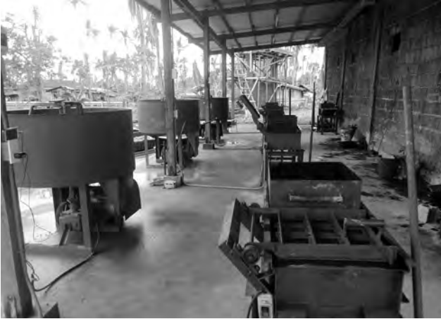
Figure 4. Machines for producing hollow concrete blocks that will be sold to agencies involved in the reconstruction of other cities. Javier, Leyte. Photo: by the author, March 12, 2014.
