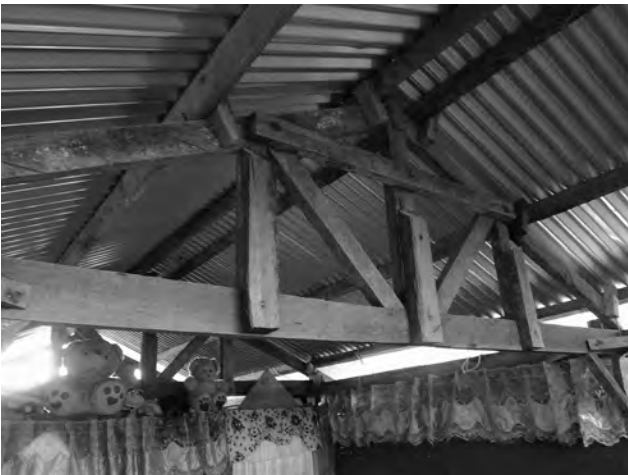
Figure 7. Interior of temporary amakan (bamboo) shelter provided by CRS showing poor construction skills in the coco lumber roof framework in Caparas an Guti, Palo, Leyte. Photo: by the author, March 13, 2014.
