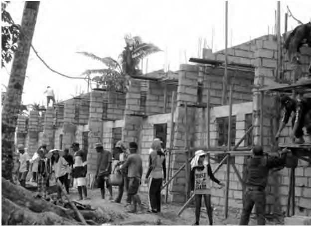
Figure 8. Users are involved as unskilled labor to pass or carry construction materials in Tanauan Leyte. Photo: by the author, March 11, 2014.
