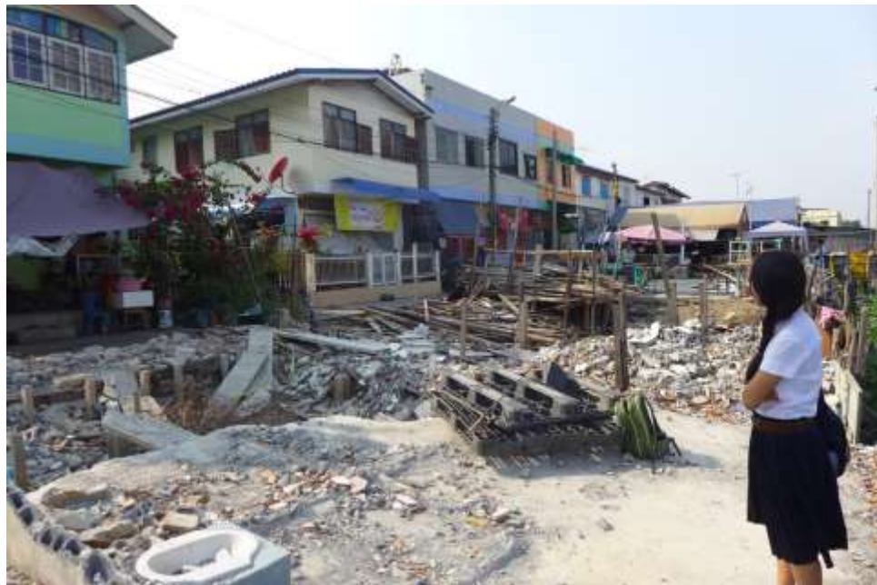
Figure 8.1.a: Saphan Mai in the process of reblocking and reconstructing the last phase of houses. Source: the author
