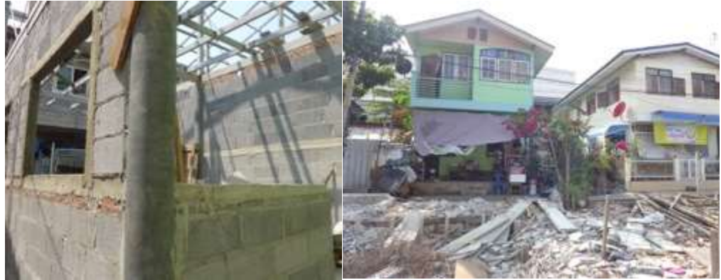
Figure 8.5.1b: Homes less vulnerable to the floods were the ones that were constructed from a mix of concrete, wood and brick as shown in the photo of a house frame on the left. Less vulnerable homes have two stories as shown in the photo on the right. Source: the author
