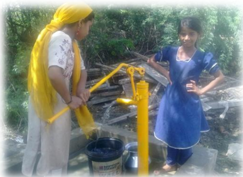
Figure 3: Hand pump installed by Tearfund WASH team in UC Jaar
