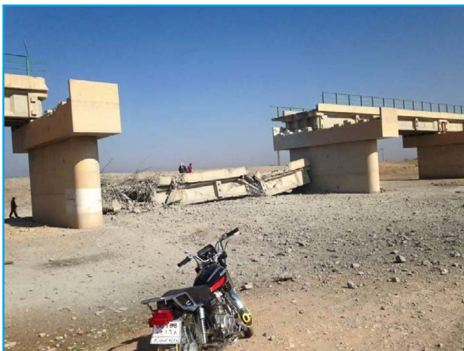
Damages at Sekkat al Qetar Bridge following an attack by fixed-wing international coalition warplanes – March 6, 2017
