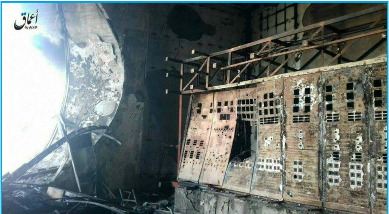
Damages in the main control room at Euphrates Dam in Raqqa suburbs following at attack by fixed-wing international coalition forces warplanes – March 25, 2017
