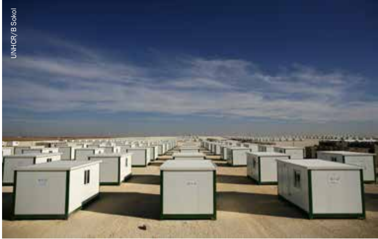
Thousands of new pre-fabricated homes being installed in Za'atari refugee camp in preparation for winter. 2012.
