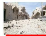
Category 4 (Destroyed) *In addition to previous categories Unusable houses or building leveled Repair not possible
