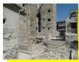
Category 2 (moderate damage) *In addition to light characteristics Under 30% roof damaged Severe fire damage Repair possible
