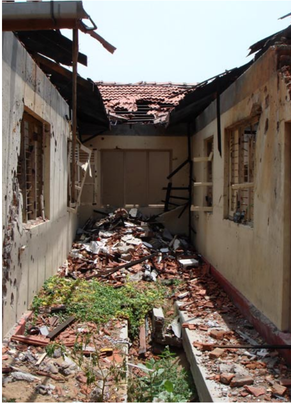
A war damaged hospital building.
