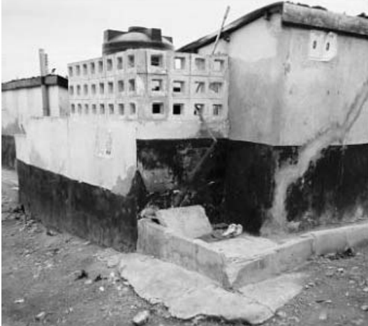
Figure 4: A poorly maintained public latrine on the outskirts of Maamobi, Accra.
