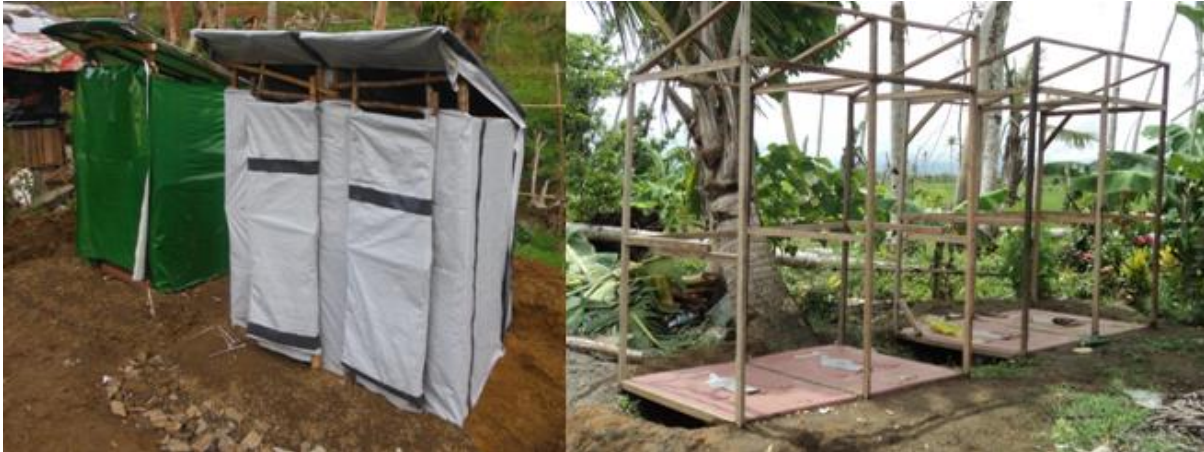
Photo 2: Communal toilets provided during the emergency phase and at present still implemented by some WASH Partners
