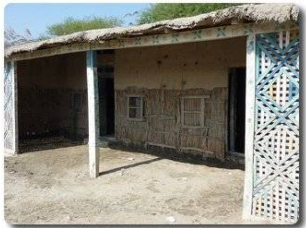
Illustration 2: House damaged by slow rising water
