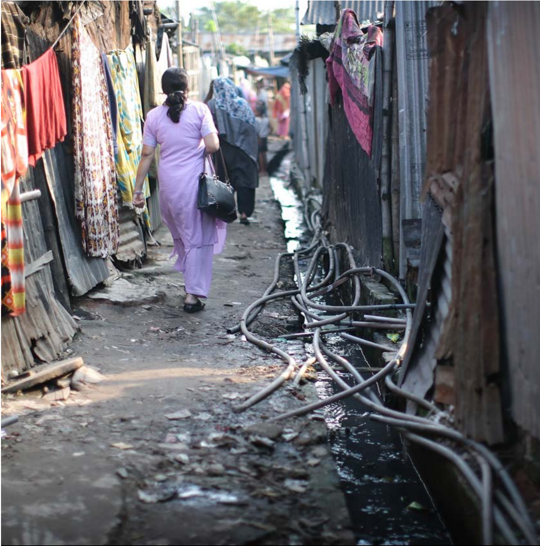
A tangle of pipes supplies water to unofficial water points in the Korail slum in Dhaka, Bangladesh.
