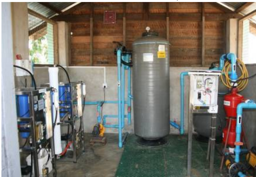
The water purification plant
