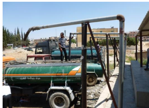
Photograph 2. Water trucking hydrant in Zarqa, Amman, Jordan 3
