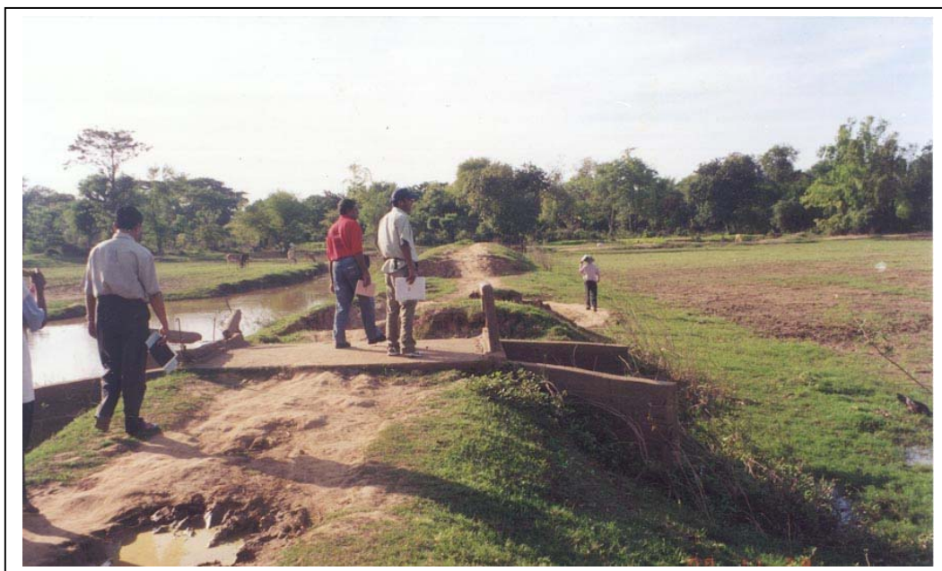
Flood damage to project road in West Prasath (Prasath Lek), in Prey Veng.
