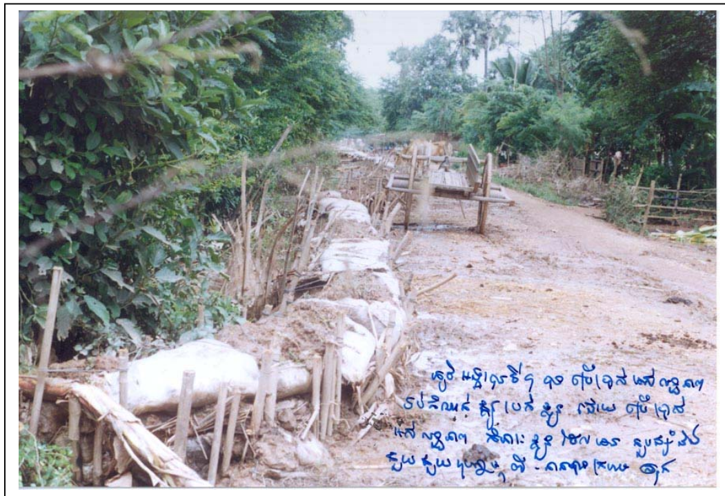
Flood barrier built from sandbags and bamboo sticks in Kang Meas district, Kampong Cham, with the assistance of the District Red Cross officer.
