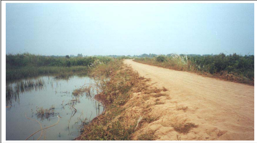
The flood mitigation project road in Prek Cham, Prey Veng has been repaired to pre-flood conditions.
