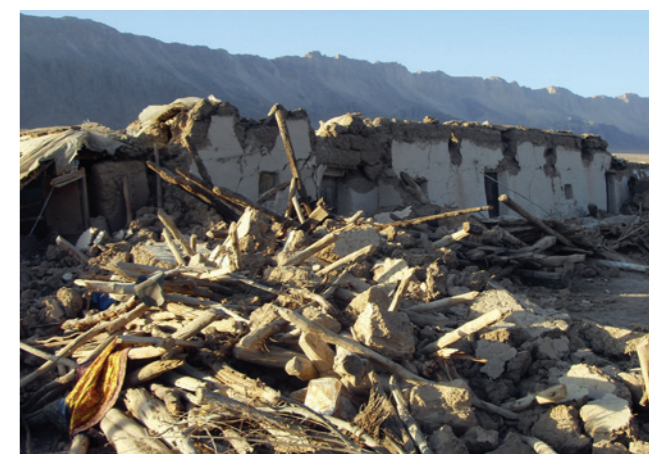
2008, Ziarat, typical mud wall long house, fully destroyed.
