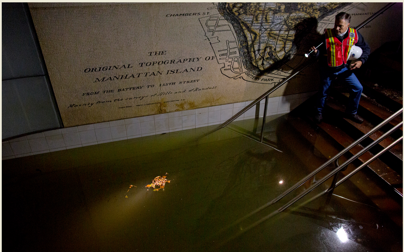
Joseph Leader, vice president and chief maintenance officer of the Metropolitan Transportation Authority, shines a flashlight on standing water inside the South Ferry 1 train station in New York, 31 October 2012. Subway stations and tunnels throughout Lower Manhattan were flooded by Sandy's storm surge. A portion of the Community Development Block Grant Disaster Relief funds authorized in January 2013 will go toward investments in infrastructural resilience against future disasters. © AP Photo/Craig Ruttle
