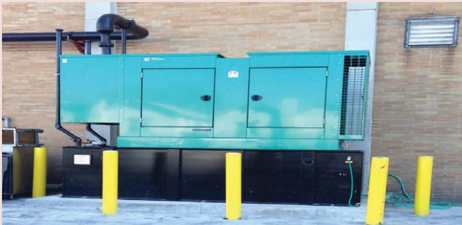
At Shore View Nursing Home in Brighton Beach, an emergency generator was moved from the basement and elevated on a raised platform.
