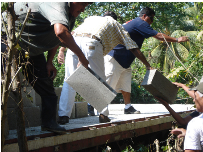
At a central point within the community, family members of 16 beneficiary households in Santa Ana Mixtan unload materials ordered through the voucher catalog. Families used the materials to repair their homes after heavy flooding. Lauren Young/CRS
