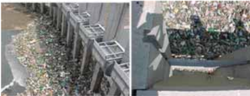
Figure 3.8. Refuse accumulating in drainage (São Paulo - Brazil)
