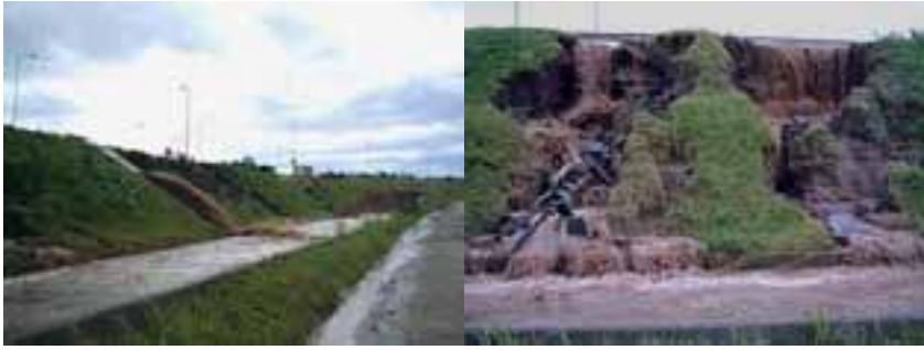
Figure 6.27. Damage to the outer canal during the storm of December 2003. Situation before and after the peak of the flood.
