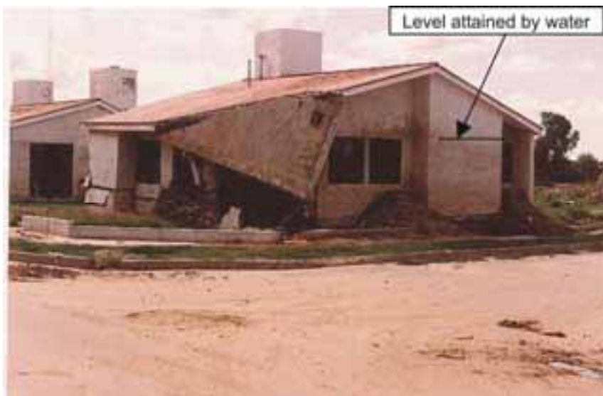
Figure 6.44. Damage to dwellings in a district of San Carlos Minas, Argentina. Flooding, January 1992.
