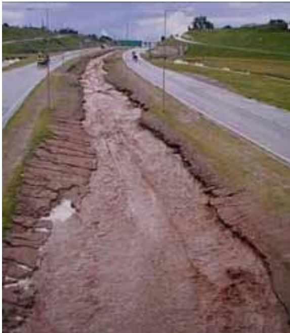
Figure 6.30. State of the central canal of the north-east section during the storm of December 2003.
