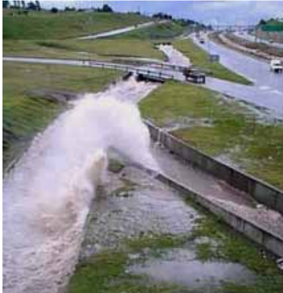
Figure 6.29. The inner canal during the storm of December 2003. Note the effect of the poor hydraulic design of the transition.
