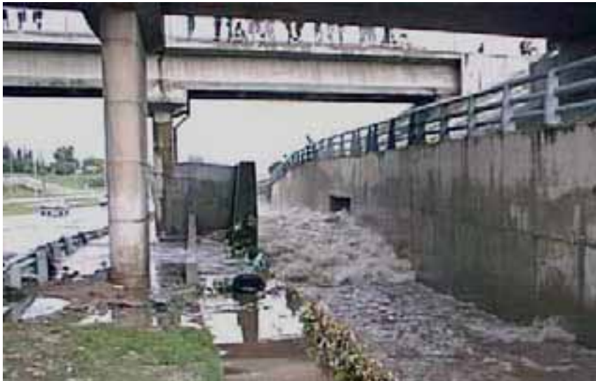
Figure 6.28. The inner canal overflowing during the storm of December 2003.
