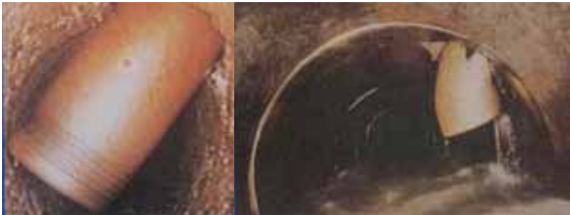
Figure 6.55. Pipes discharging directly into the storm drains. (Source: Cruz and Molina, 2004).
