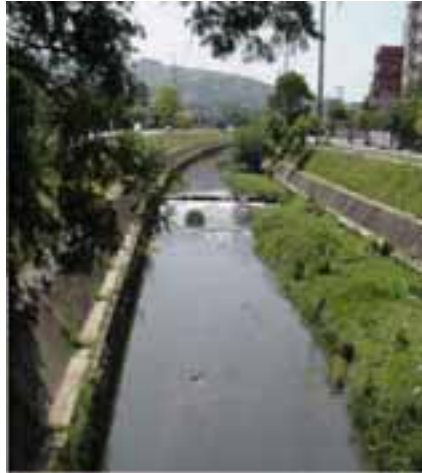
Figure 3.9. Obstructions to flow in canals (Porto Alegre, Brazil).
