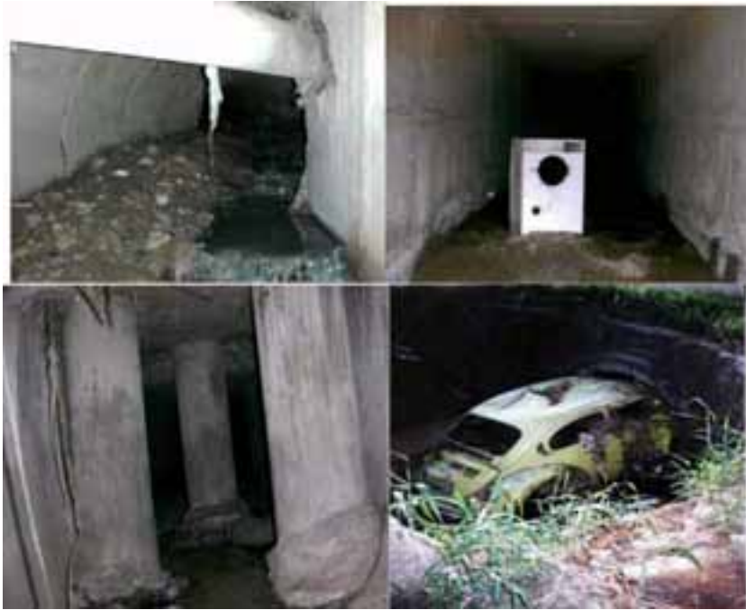
Figure 3.7. Obstructions and refuse in the drainage (Belo Horizonte and São Paulo – cities in Brazil)
