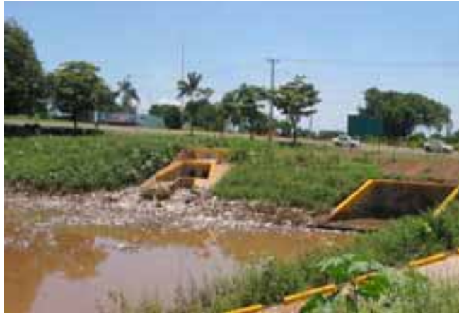
Figure 6.64. Concentration of urban refuse in the Los Gauchos Tiscapa micro-dam, opened in 2005. City of Managua.
