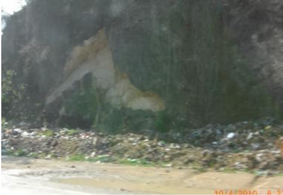
Figure 5.2: Slip failure in a cutting next to the highway
