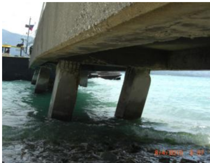
Figure 4.16: A view of the underside of the wharf showing the damaged piles
