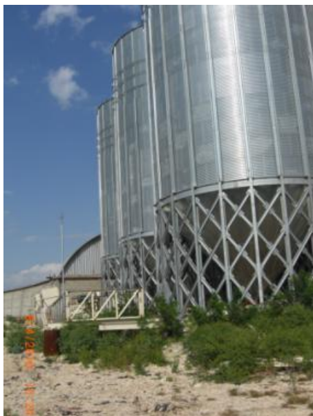
Figure 4.19: Silo structures that are undamaged with building with collapsed roof in the background
