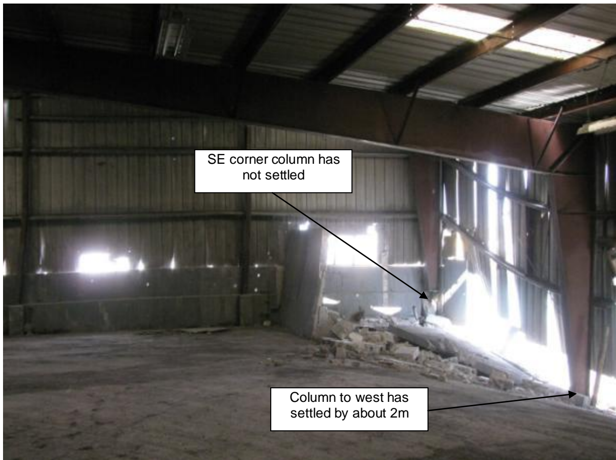
Figure 7.5: Settlement of columns in SE corner of warehouse
