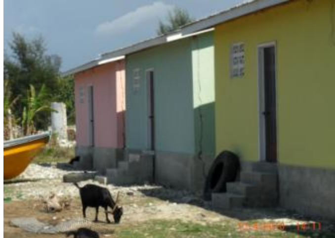
Figure 4.21: Damaged houses displaying extensive cracking
