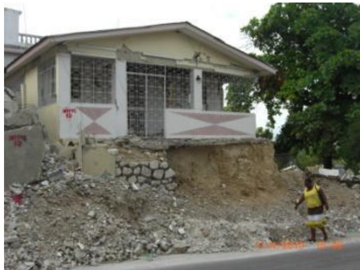
Figure 8.6: Damage to a house in location L at the top of a 10% gradient hill
