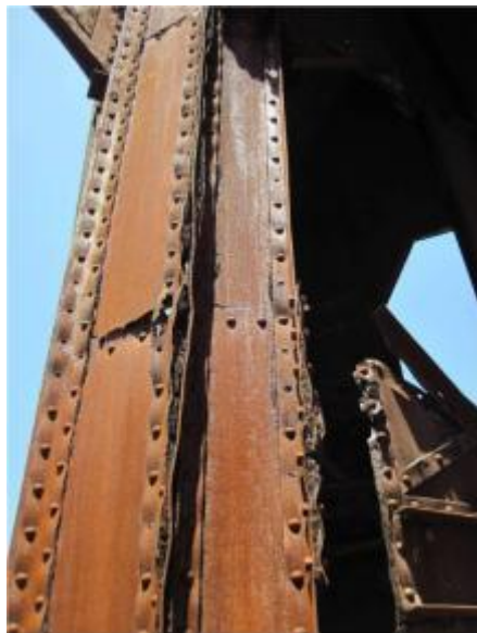
Figure 7.9: Corrosion of a column in the clock tower
