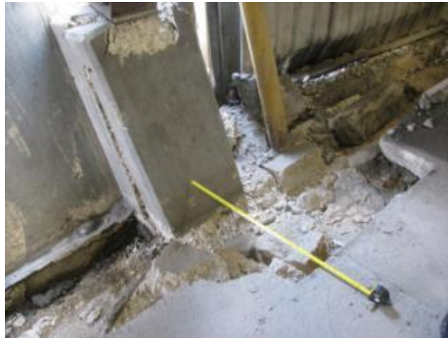
Figure 7.3: Lateral and vertical displacement of warehouse foundation
