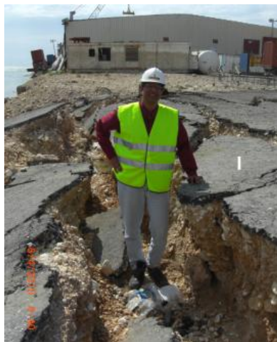
Figure 4.10: Cracks induced by lateral spreading close to north wharf extending to a depth of about 1m
