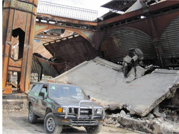
Figure 7.11: Failure of concrete canopy adjacent to north west corner of south market
