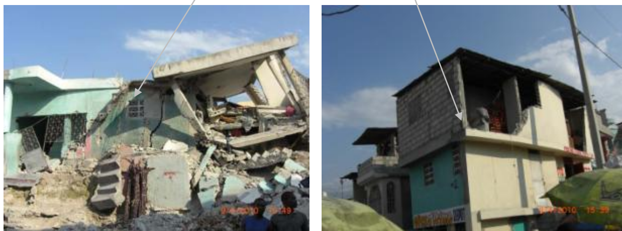
Figure 6.24: (left) Completely collapsed building. Both GEO-CAN and Pictometry interpretations considered this building to be two separate buildings. (right) Heavy damage to infill wall on the third storey. This type of damage often cannot be seen from above.
