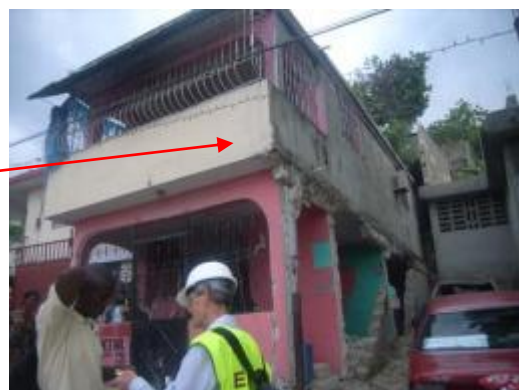
Figure 6.21: Building with serious damage to the infill wall on the ground floor.
