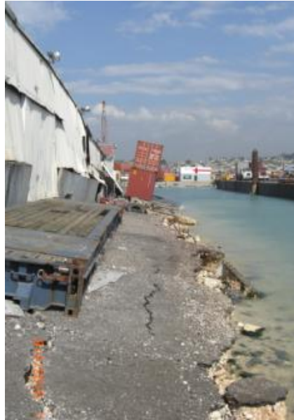
Figure 4.11: Collapsed Section of the north wharf
