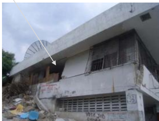
Figure 6.15: Building (b) which was assigned D4 by EEFIT. The same building looks intact in the aerial photograph in Figure 6.13. Pictometry and GEO-CAN assigned D1 and D0, respectively.
