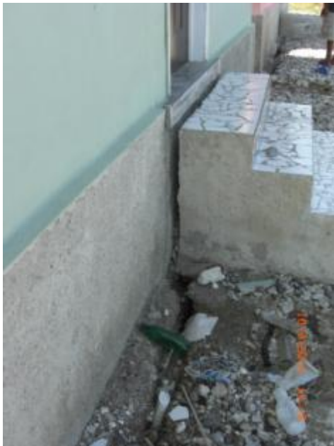
Figure 4.23: Close-up view of the steps that separated from the buildings
