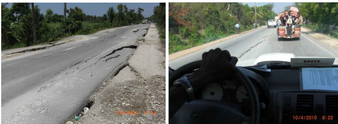
Figure 3.10: Road failure at two locations of the road between Léogane and L'acul
