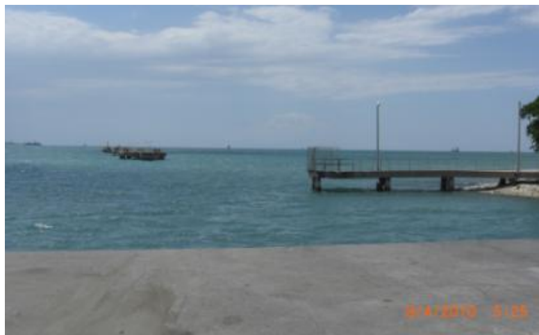
Figure 4.8: Collapsed sections of the south pier
