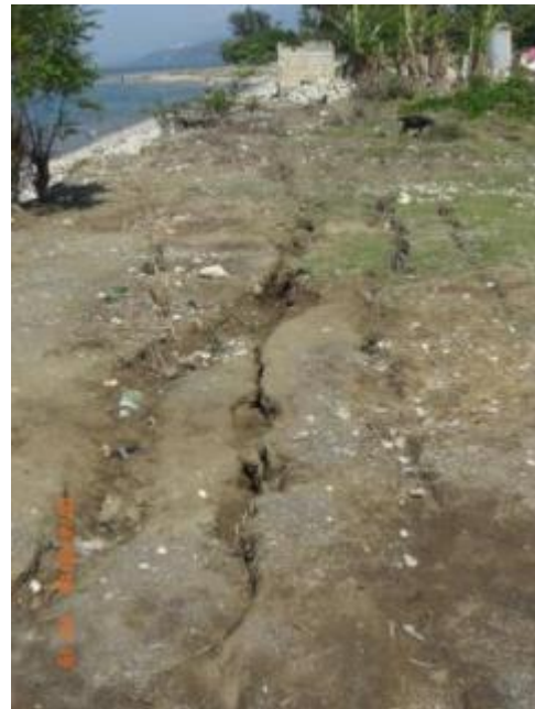
Figure 4.24: Lateral spreading continuing for some distance from the building site
