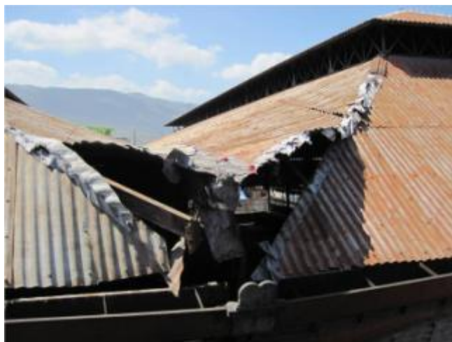
Figure 7.10: Corrosion around roof valley in south market
