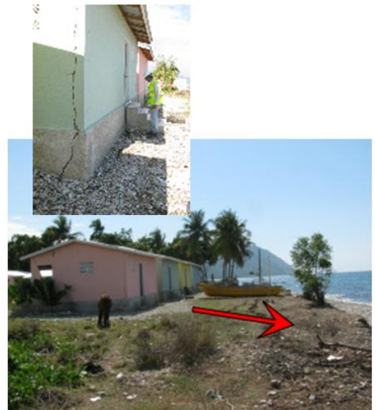
Lateral spreading has dragged forward the front of these buildings
