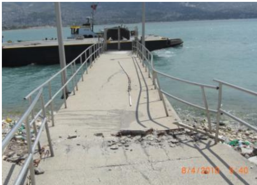
Figure 4.15: Severe damage to a pile supported wharf structure
