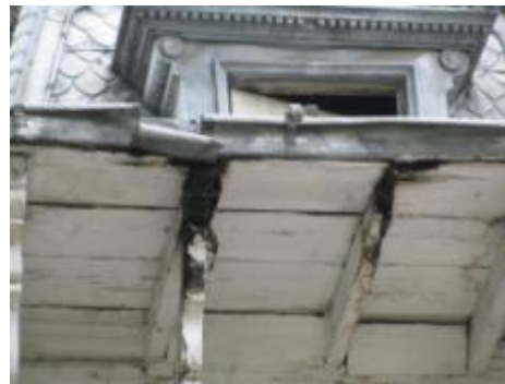
(b) Detail showing poor maintenance
