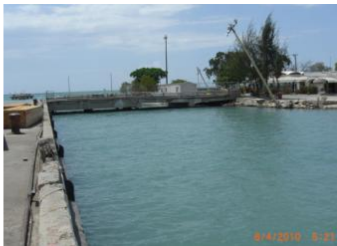
Figure 4.12: An overview of the connecting bridge linking the south pier and the island
