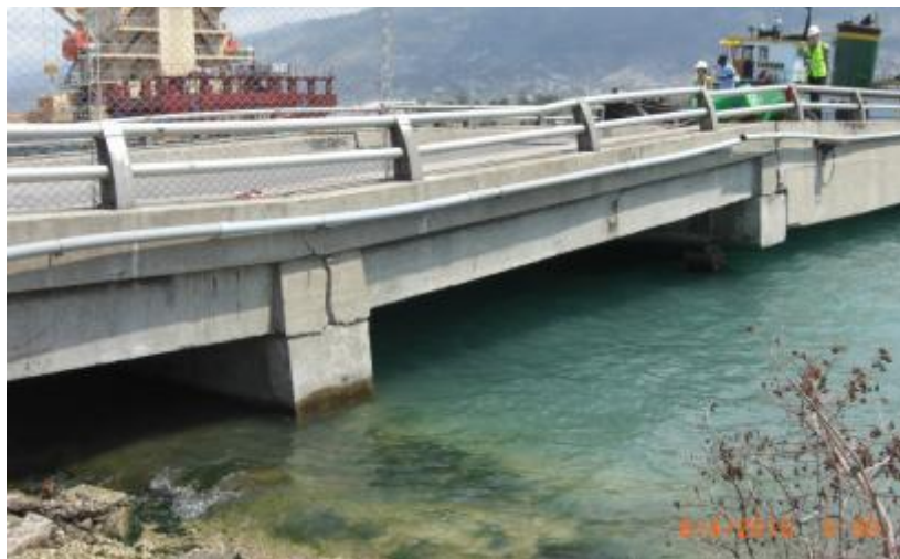
Figure 4.14: Settlement of pile foundations causes self-articulation of the connecting bridge
