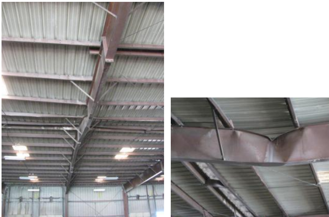
Figure 7.4: Buckling of warehouse roof beams
