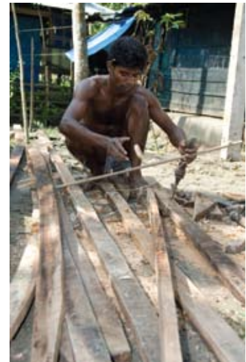
A worker uses a hand drill to prepare beams for roof support at a CRS building site in southern Bangladesh.
