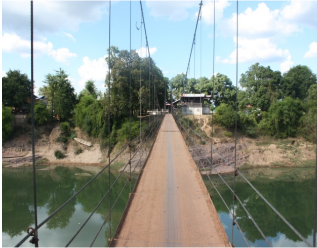
Figure 6 The bridge over Xe Bang Fai River (Nam Xe River) (By permission of J. E. Rigg 2012)
