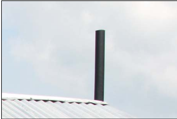
Picture 12. Kitchanga primary school has a well constructed 6 cubicles toilet, but the vent pipe is not covered with a fly screen
