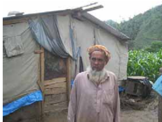
Figure 10: Deteriorating temporary shelter after 9 months occupation
