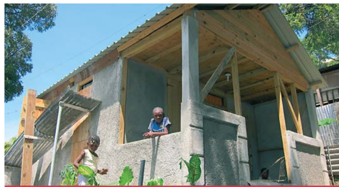
A new safe permanent housing model – together with the local Haitian authority, the Affordable Housing Institute and the Foyer Sainte Marie, Cordaid is introducing this new housing model in Port-au-Prince.
