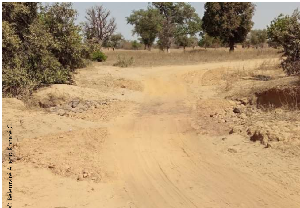
Figure 5. Rehabilitation of a track through the “Cash for Work” modality in Koulogo, Centre North Region, Burkina Faso
