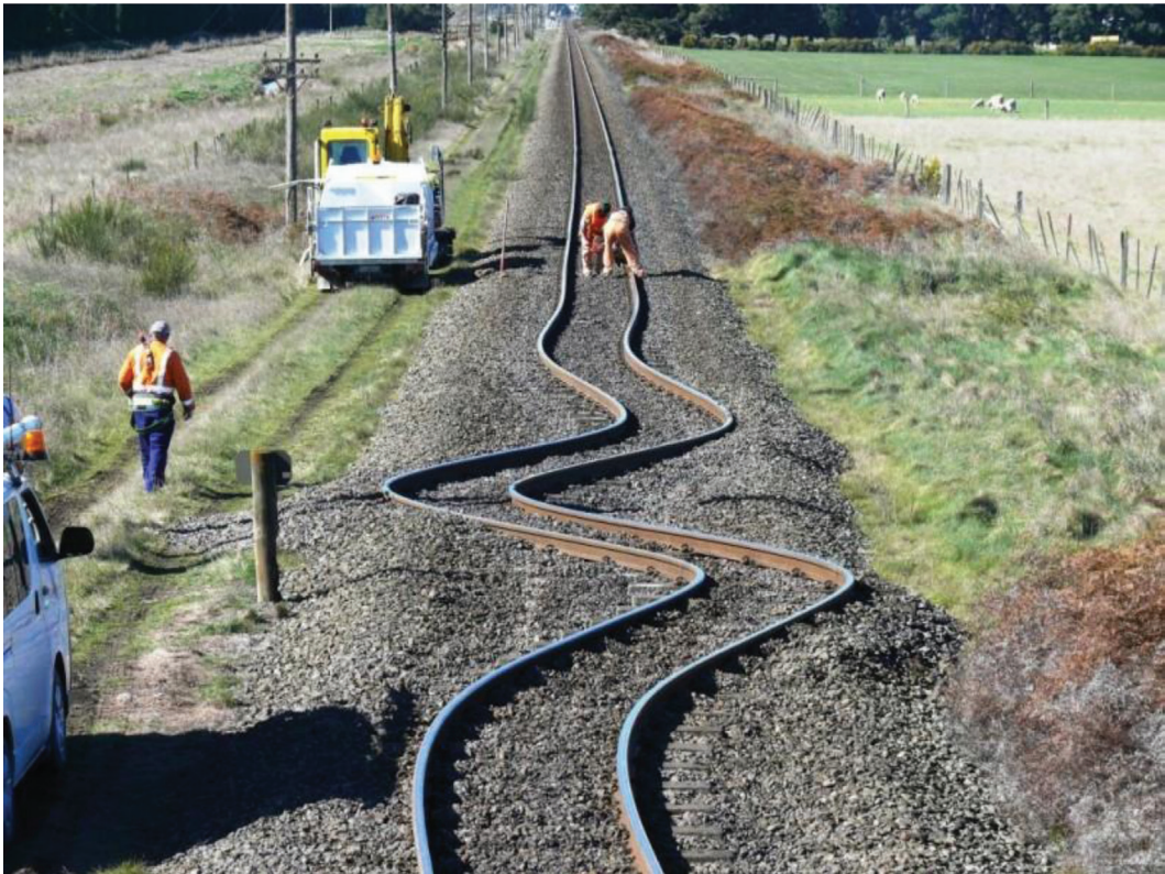
Figure 3.4 A New Zealand Railbed after an Earthquake
