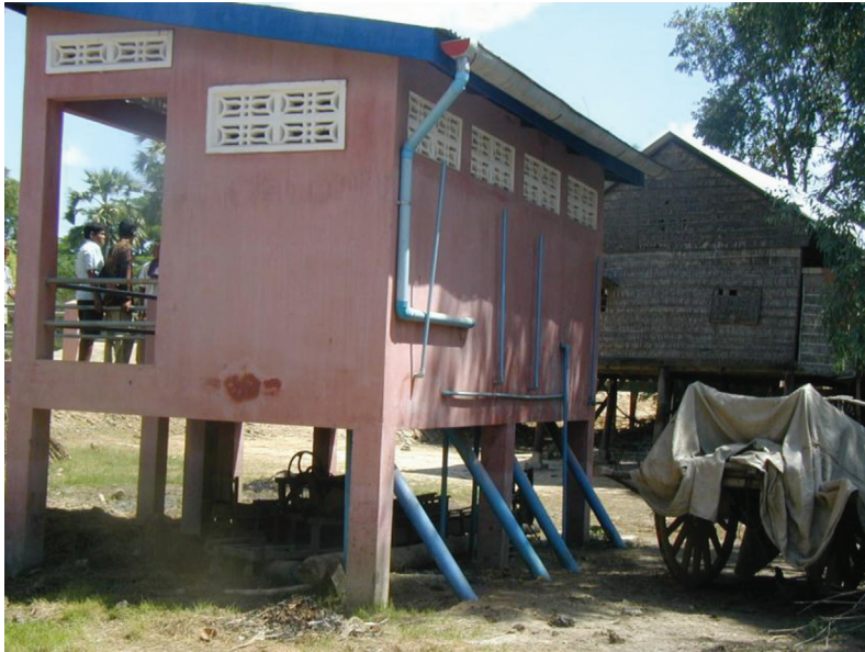
Figure 3.2 Mitigation Infrastructure: Communal Toilets Elevated Against Flooding, Cambodia
