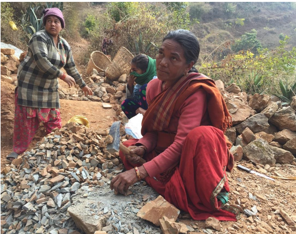
Women in Panchkhal, Kabhre, working on the reconstruction of the water supply system damaged by the 2015 earthquake. Photo: Ashim Poudel/KIRDARC.
