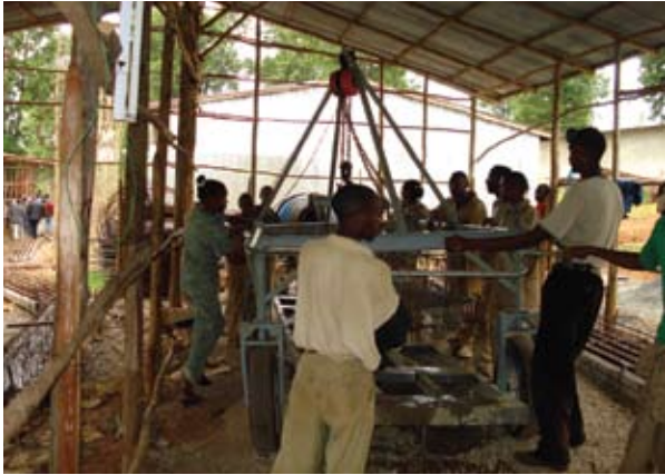
Youth groups organised under small-scale enterprises have received skill development training and are producing pre-cast beam for condominiums built under the Integrated Housing Development Programme, Yirgalem, 2007.
