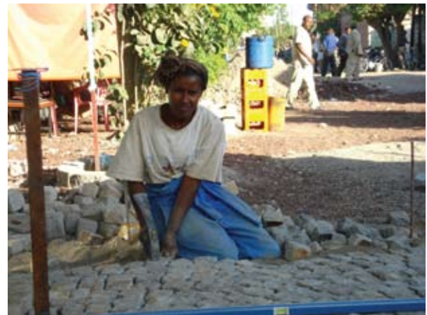
Small firms are supported to engage in municipal infrastructure and service delivery: a young woman engaged in cobblestone pedestrian road construction, Adama City, 2007.
