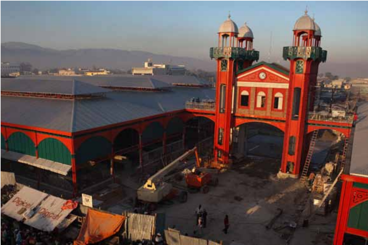
Fig. 18 The market after being rebuilt. This was paid for by Digicel, Haiti's main mobile phone operator (Reitman, 2011). Image: (John McAslan and Partners, 2011b)
