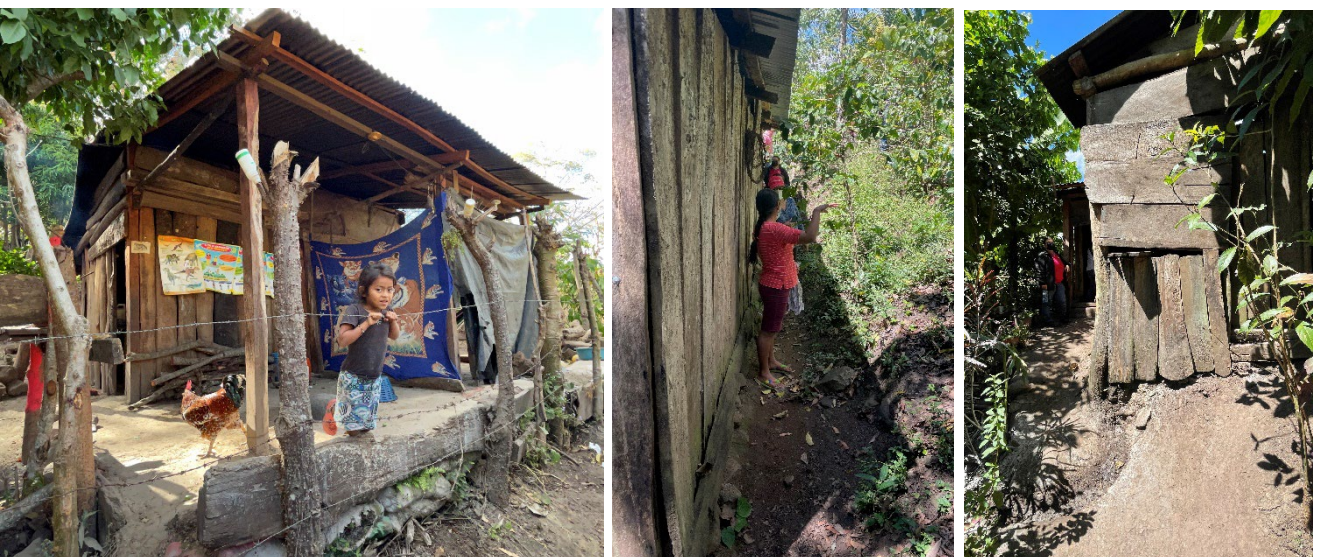
Many houses are not disaster resistant. Simple improvements as drainage or bracing could enhance their resistance
