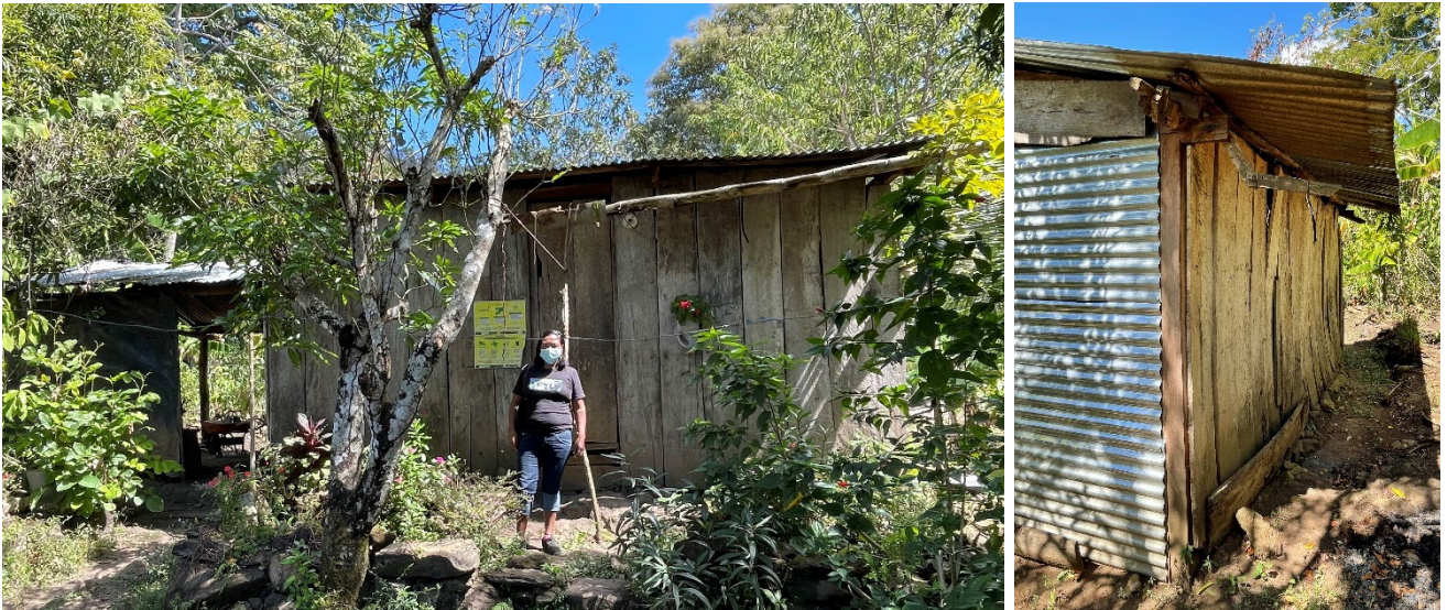
Wood could often be reused from the former house; the zinc laminates sometimes also served to protect the exposed wall
