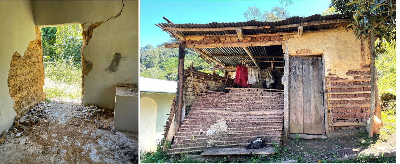
Typical damages to local buildings. Several buildings were also completely destroyed
