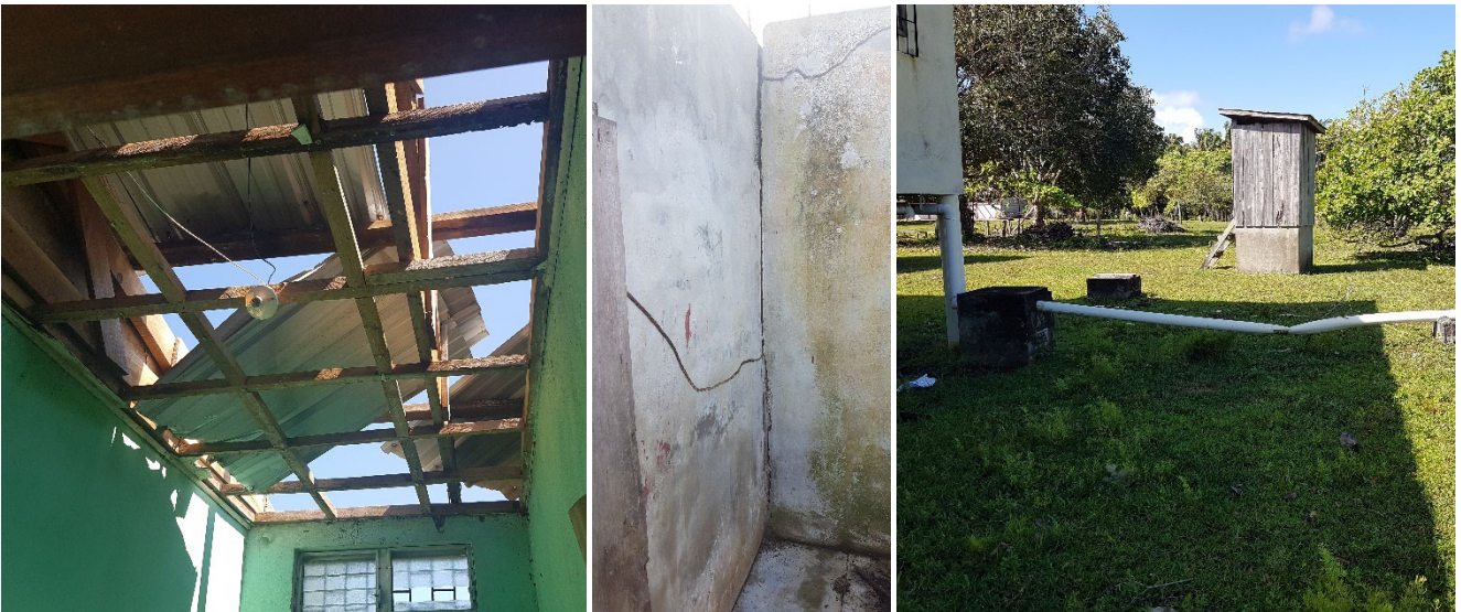
Damages to buildings (roofs, walls, windows & doors) and water supply systems (rainwater harvesting, water tanks, pipes.)
