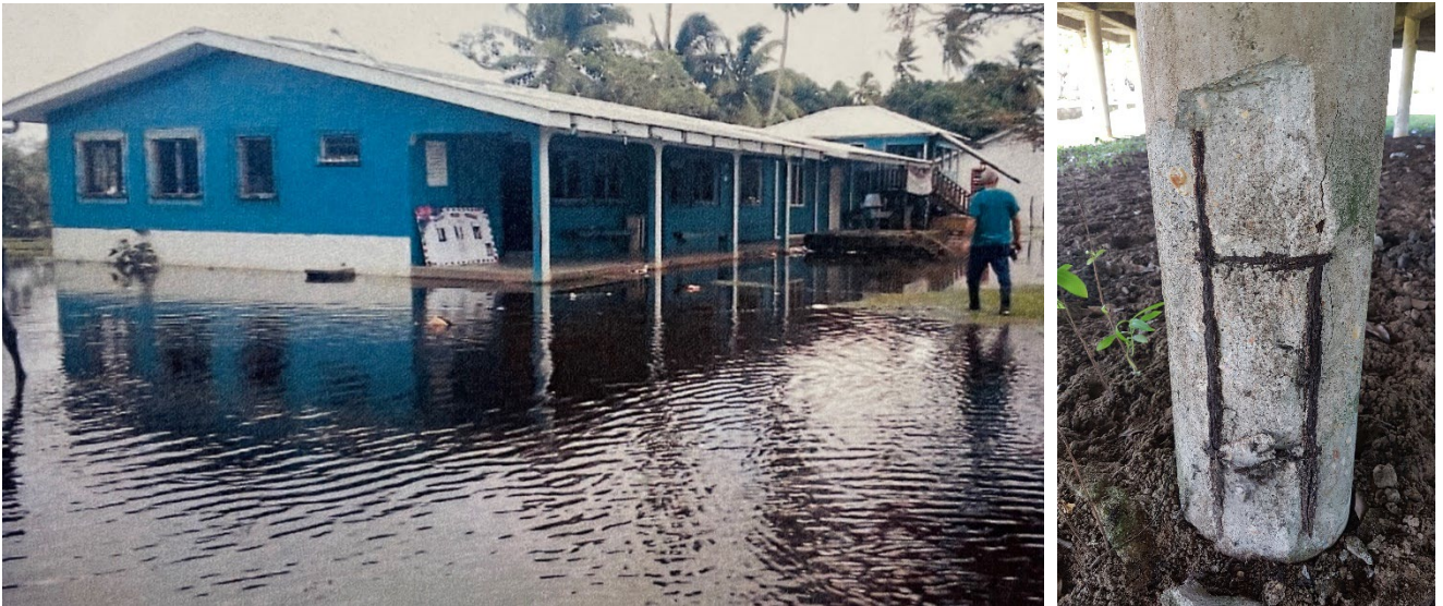
Situation: floods & high winds due to hurricanes and pre-vulnerabilities of structures due to lack of maintenance
