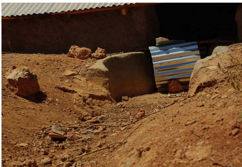
Poorly constructed inlet at a Berkad in Puntland; without the technical capacity in critical areas such as water and sanitation, the performance of relief efforts by the national society will suffer.
