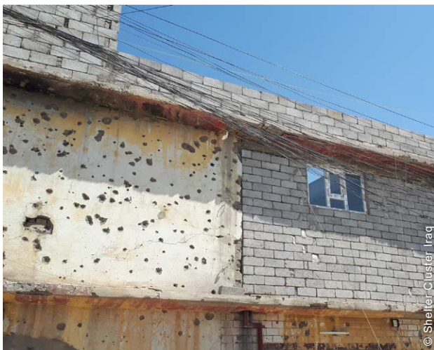
Since the end of the conflict, damage and destruction of housing is one of the key barriers to displaced people being able to return.
