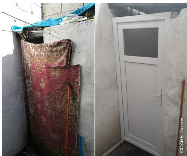
Before and after: Installing doors to improve protection, security and weather-proofing was a priority intervention.
