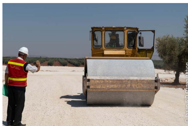
Site improvements at IDP sites included improving accessibility and reducing flood risk.
