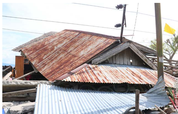
The project involved multiple components, including rubble removal support to help with the clearing of family plots.
