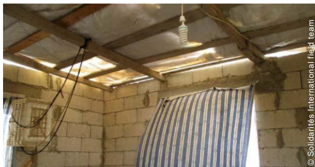
Many houses had previous makeshift repairs carried out, such as this improvised roof.
