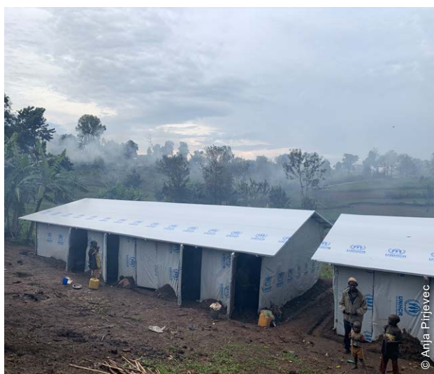
79 collective shelters were built in host communities to support IDPs sleeping in the open air or in public buildings. Collective shelters were partitioned with separate units for eight households.
