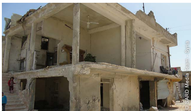
Many IDP, returnee and vulnerable local households were living in significantly damaged homes.
