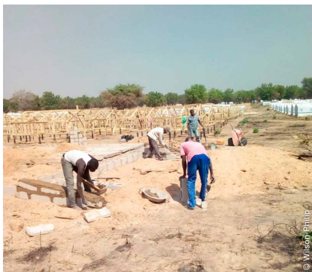
Shelter and latrine construction commenced in October 2017 in preparation for the anticipated relocation date of January 2018 (which was later brought forward to mid-December 2017).
