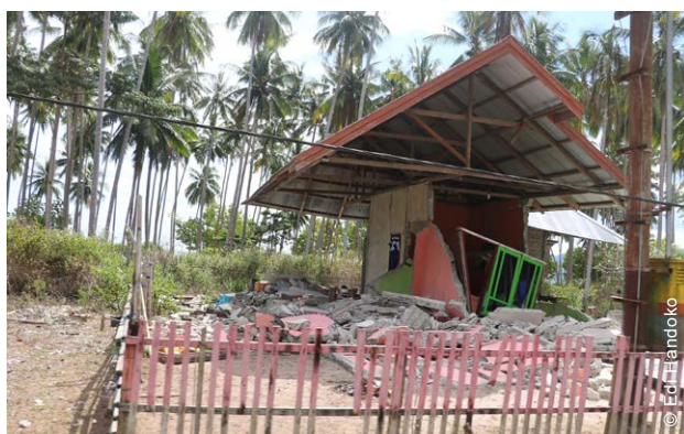
Following the earthquake, 90-95% of homes in Lombonga were severely damaged or completely destroyed.
