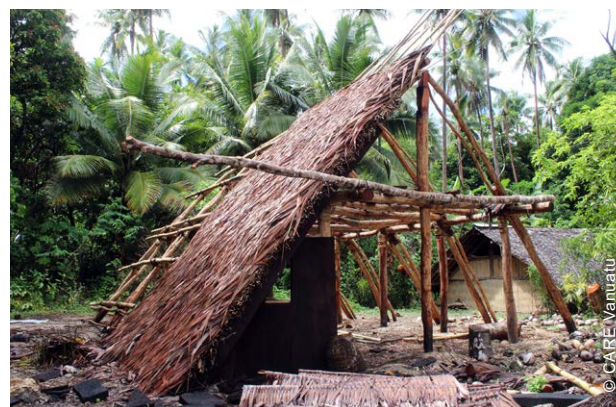
Model house structures were built at the community level on Maewo, to demonstrate traditional safe construction principles for all shelter training and awareness activities.
