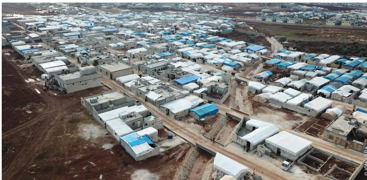
A variety of interventions were carried out based on the needs and technical assessments of each camp. These included constructing open and closed drainage systems, sewage systems, culverts, roads, and raising tents 20cm off the ground through graveling.
