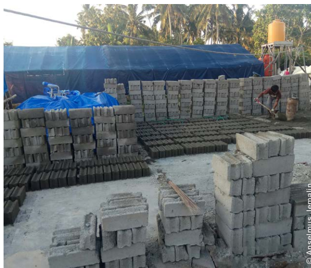
The project engaged local suppliers as much as possible for the production of materials that could be made locally, such as concrete blocks, doors and windows.
