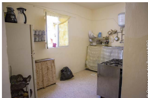
One priority for renovations was to ensure separation of kitchen and bathroom spaces. Here a new wall has been installed to separate the two rooms.
