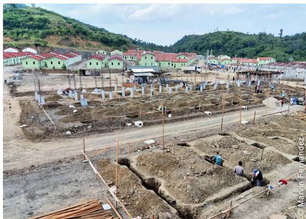
Housing construction was carried out by local contractors, with oversight and quality control from the organization's construction team.
