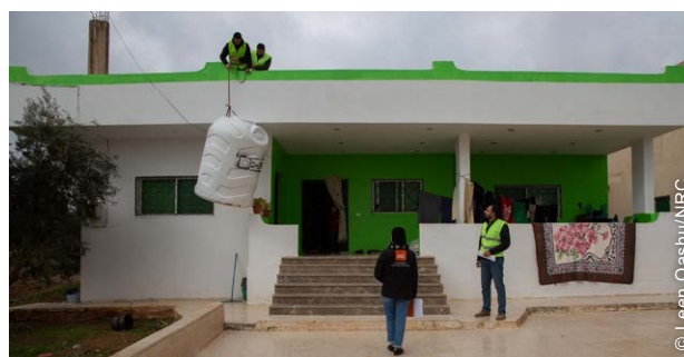
WASH rehabilitation conducted as part of the program, included the installation of water tanks.
