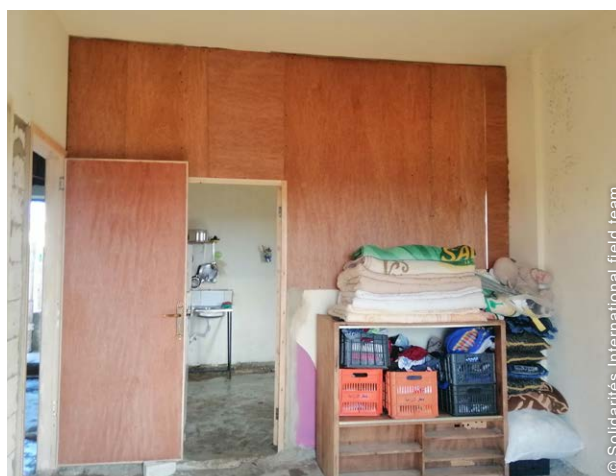
Partitions were installed to separate the kitchen from the living/sleeping space. This improved hygiene and allowed more privacy.
