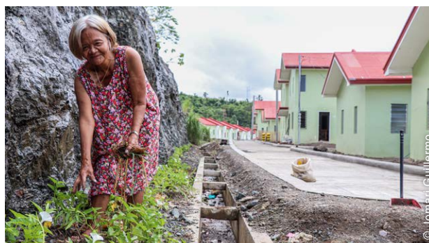
The project supported households to obtain their land title through either grants, cash payment, or loan.
