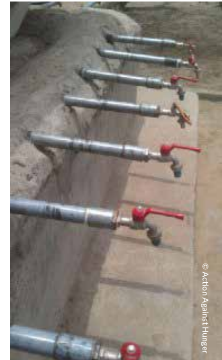
New water allocation system in Al-Mikhraf Village
