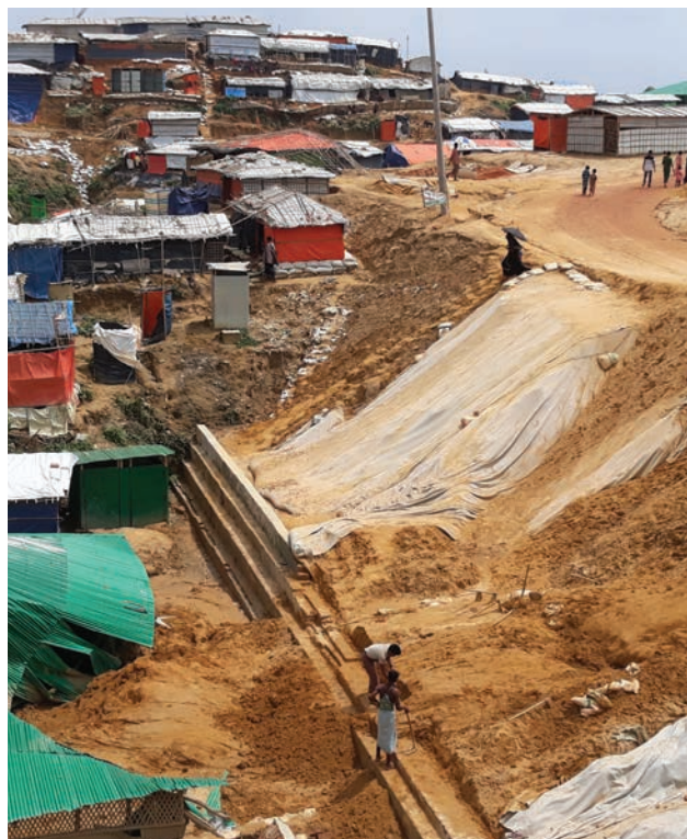
Kutupalong-Balukhali camp. After a night of torrential rain, the author arrived to see a landslide had partly destroyed a health centre.
