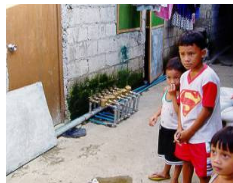
Photo 4 – Meter battery in a Manila street (Photo Maynilad)
