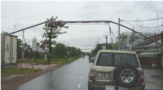
Photo 9 – Small network piping crossing over the road (Southern Vietnam)
