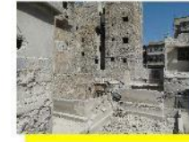
Category 2 (moderate damage) *In addition to light characteristics Under 30% roof damaged Severe fire damage Repair possible
