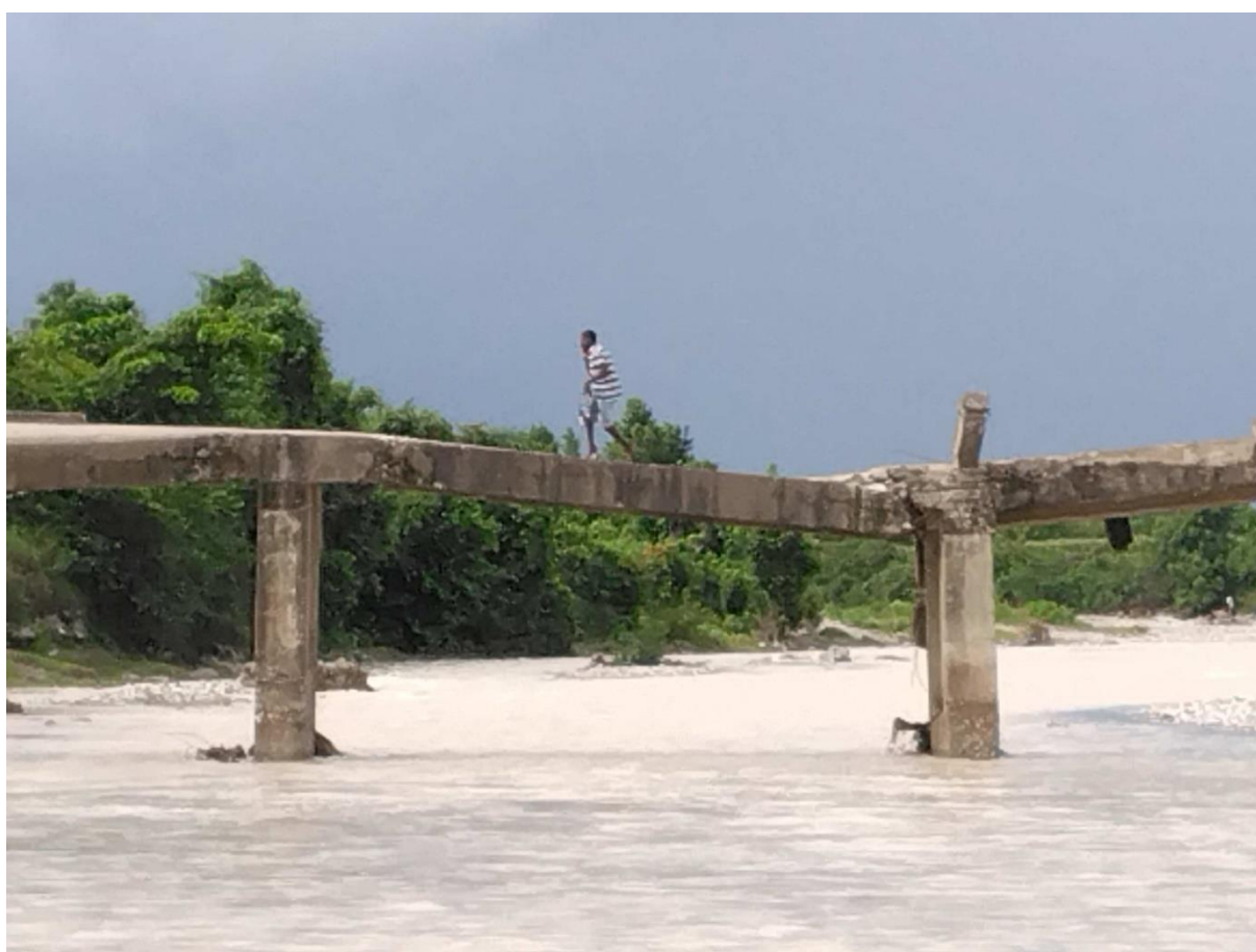
PHOTO N°6: DESTROYED BRIDGE IN THE SUD DEPARTMENT
