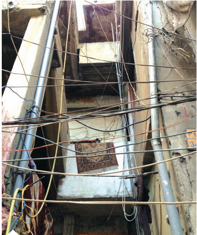
Electric cables of a building in Naba'a, Lebanon 2014. Photo © UN-HABITAT / M.Fawaz
