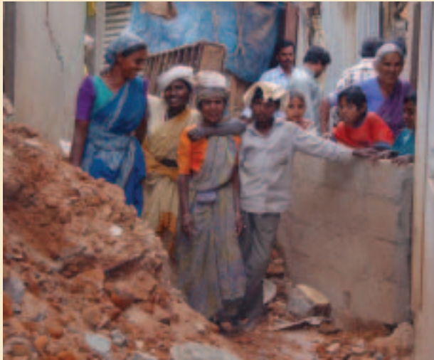
Community members involved in constructing the third housing block at Sunnuduguddu, Bangalore, India. The development at Sunnuduguddu is supported by the CLIFF programme.
