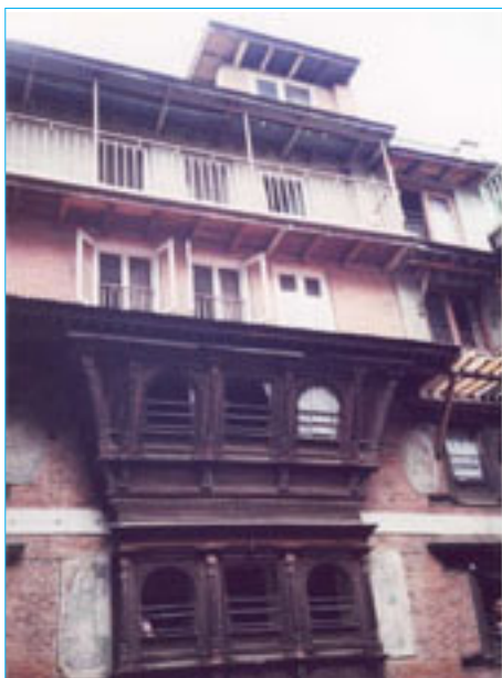
A typical Nagbahal house, which was originally two- or three-storey. Additional stories have been constructed recently, increasing the community's vulnerability to earthquake risk.
