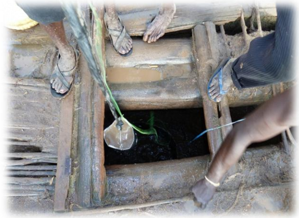
Figure 2 Hand dug well for irrigation of community gardens, Lodwar
